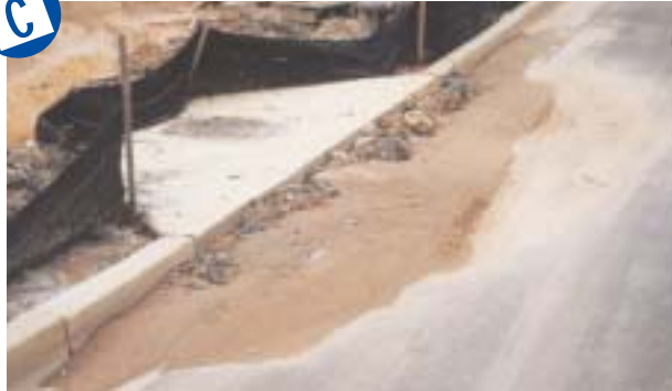
Good application, but needs to be cleaned out to function properly.
