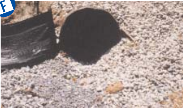
Very poor stone coverage. Entire channel should be protected.
