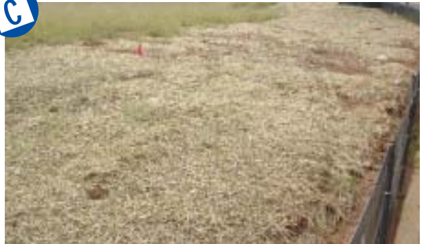
Good coverage of mulch and temporary grass, but runoff has exposed some areas.
