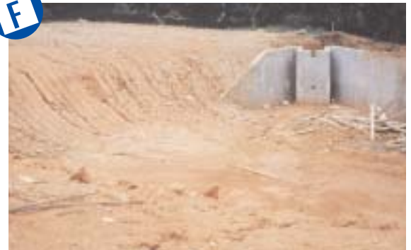
No vegetation. Perforated standpipe with gravel filter is missing.
