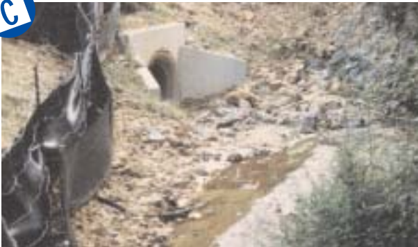
Poor geometry. Inadequate stone coverage.
