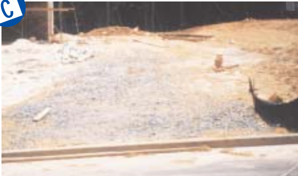
Fair stone coverage. Some mud tracking onto roadway.
