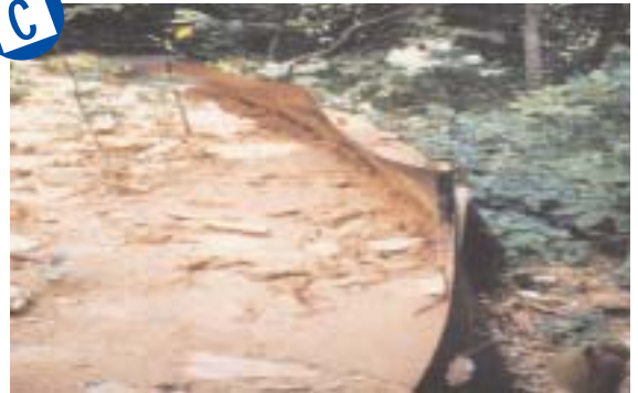
Silt fence adequate: but NEVER stack silt fences.
