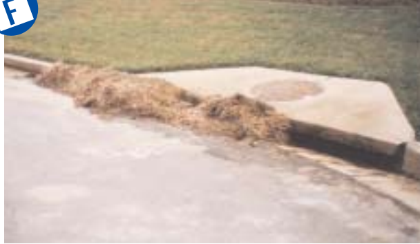
Poor inlet protection. Hay bales do not last very long. May clog inlet or pipes.
