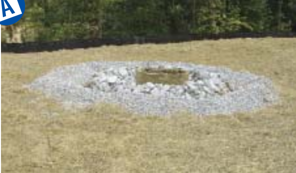
Excellent stone sizing and placement. Note: good surrounding soil coverage with mulch.
