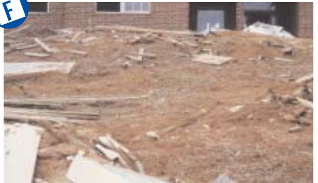
Completely inadequate coverage.
