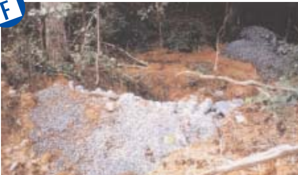
Poor application. Virtually unmaintainable without significant disturbance. Removal of feature at completion very difficult.
