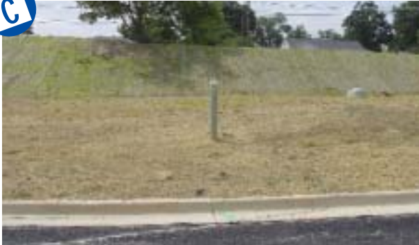
Matting applied to slopes, some areas exposed. Vegetation beginning, watering needed. Mulching in foreground pretty good.
