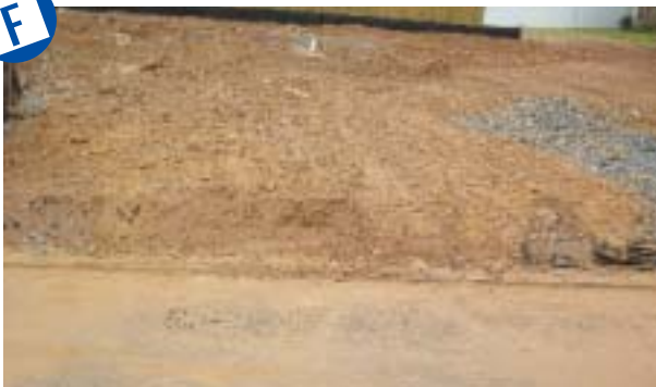
Very poor stone coverage. Significant mud tracking and flowing onto roadway.
