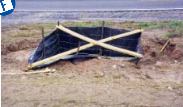
Very poor maintenance. No protection.
