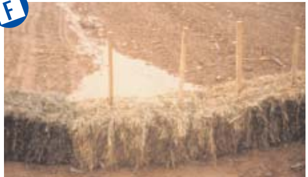
Poor application of hay bales. Not imbedded in soil. Water easily migrates under bales causing failure.
