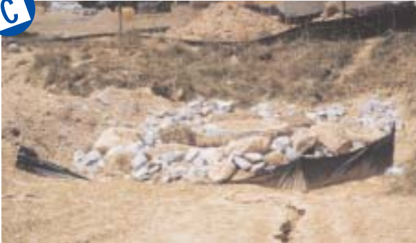
Rill erosion beginning in foreground (concentrated flow). Silt fence down. No small stone for filtering.
